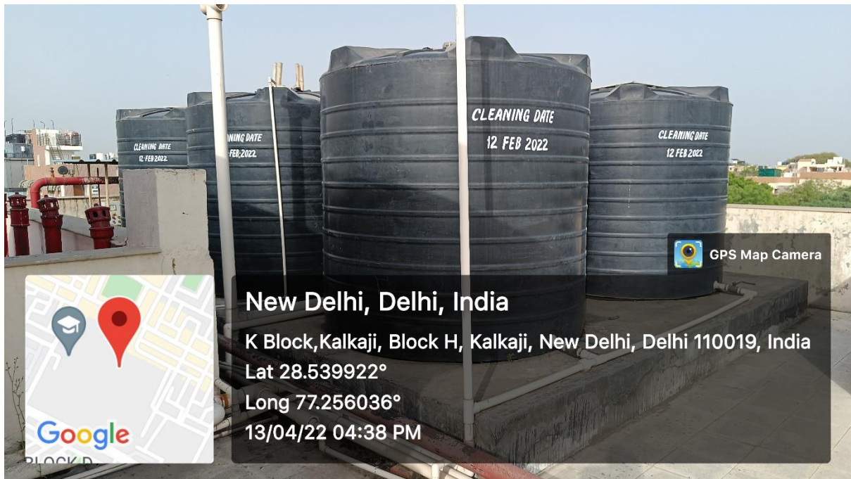
Figure.8 Water storage tanks on the new block of the campus with the latest cleaning date
