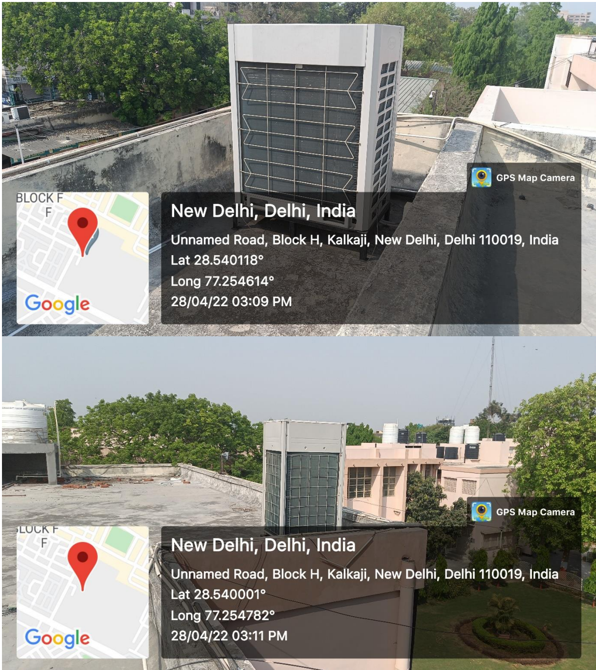
Figure.2 Various VRF units to increase energy efficiency in administrative building and new science block second floor of the college.
