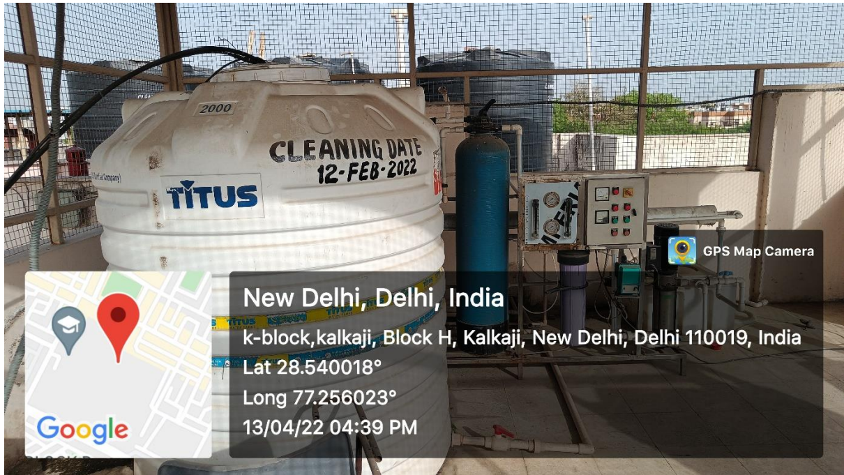
Figure.10. Reverse Osmosis water treatment system
